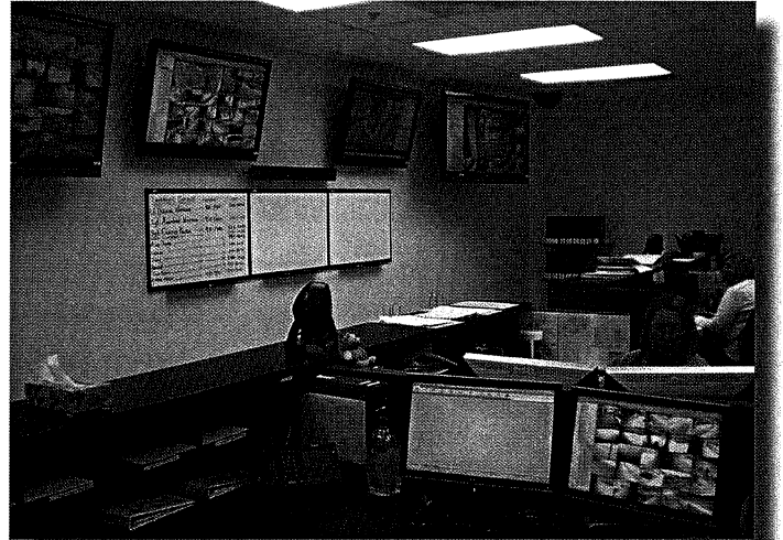
Pictured is the video surveillance monitoring station at Leon County, Florida, Public Schools.
